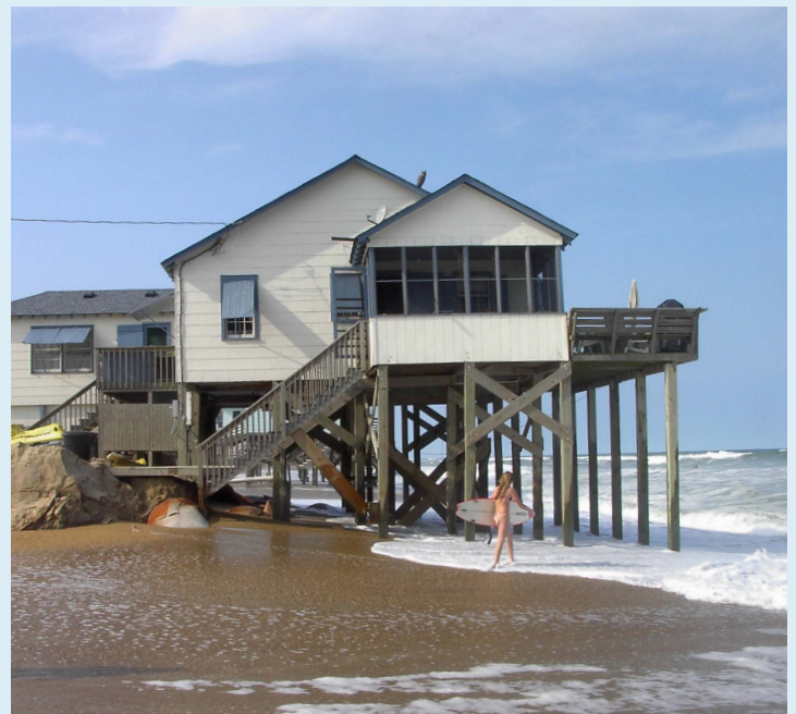
Beach houses in Nags Head are vulnerable to severe storms, flooding, and coastal erosion. © James G Titus; used by permission.
